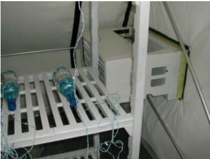
Figure 8 – Photograph of the Evaporator Inside the Cold Store
